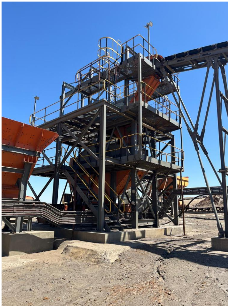
Figure 18C : NLZM Processing Plant: Screening ahead of flotation
