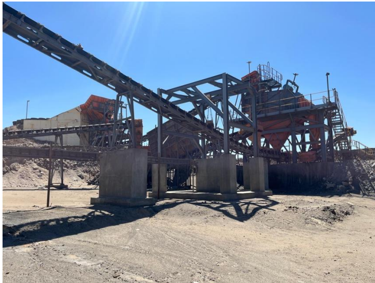
Figure 18B : NLZM Processing Plant: Primary and secondary crushers
